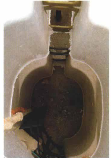
Hammering rebar into drilled holes (inset) ties wall to footing. Other methods include a keyway in the footing, L-shaped rebar cast in place and rebar epoxied into drilled holes.
