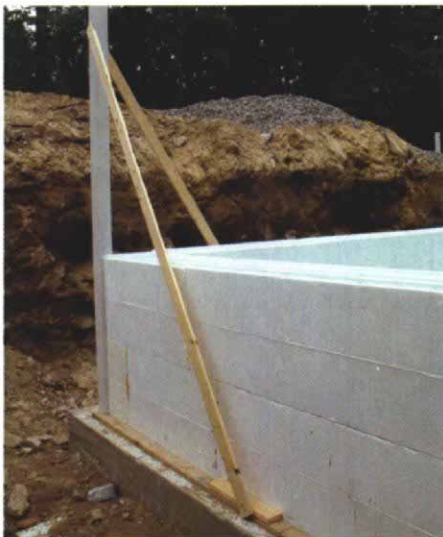
Corner braces support a relatively weak spot in the forms. Setting the braces dead plumb provides a good starting point for stacking forms.
