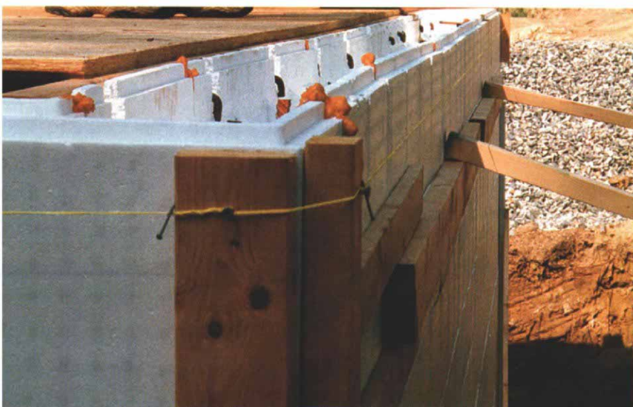
String checks walls for straightness. Tweaking the braces will bring the wall straight. If scaffolds brace your walls, your weight on them can move the walls, so stay off them while checking for straight.
